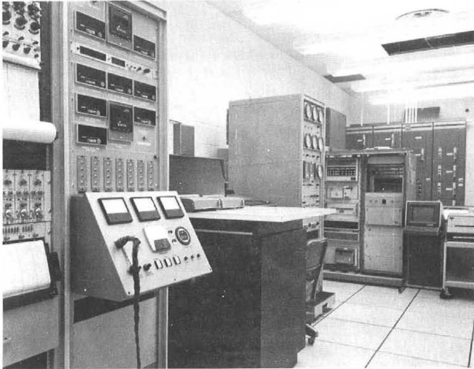
Figure 6-1. Control Room in Control and Equipment Building
