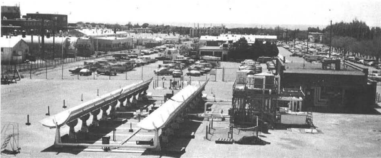
Figure 3-1. Solar Total Energy System Test Facility (collector field lower left)
