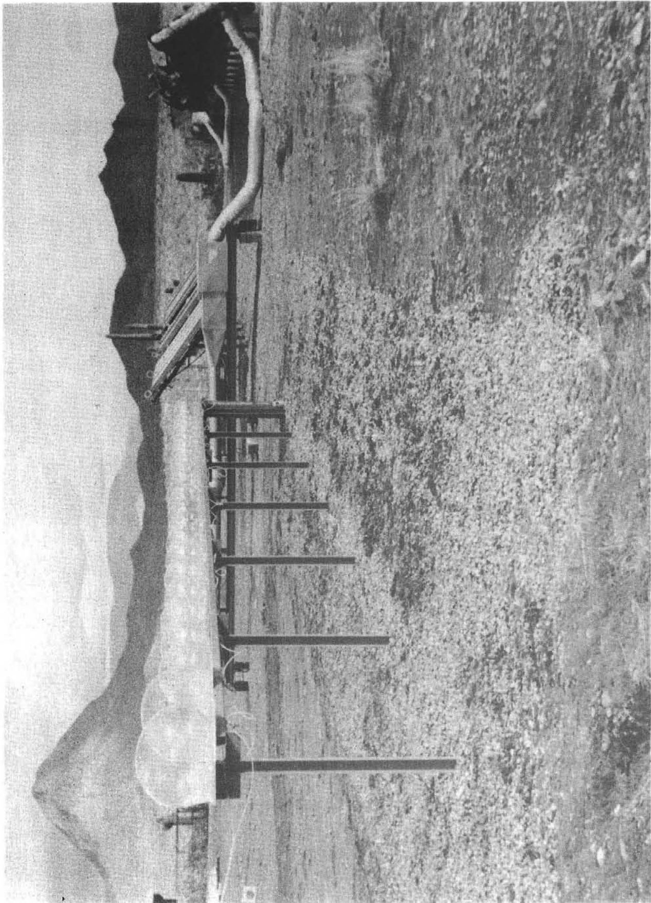
Figure 7.1-2. Photograph of Enclosures and Support Stand
