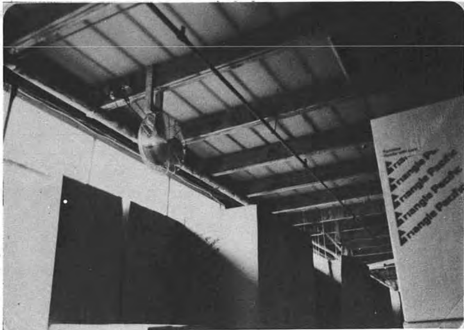
Figure 14-3. Circulating Fans in Warehouse
