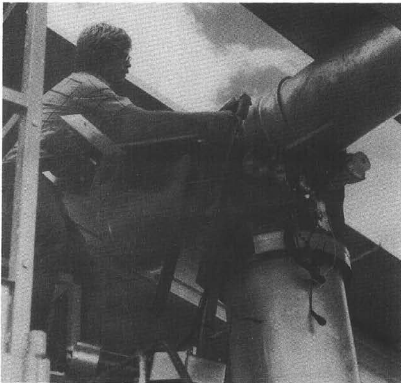
Figure A-8.2. MDAC Damaged Stow Jack Being Replaced
