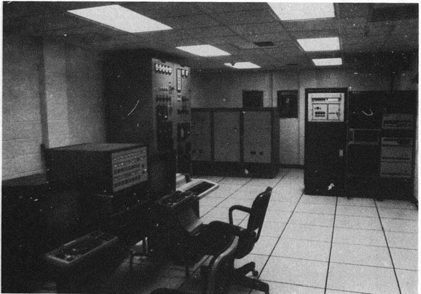
Figure 9. Control Room, Data Acquisition Center, and Switchgear
