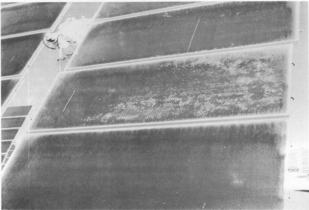
Figure 9. Photograph of Corroded Mirror Modules
