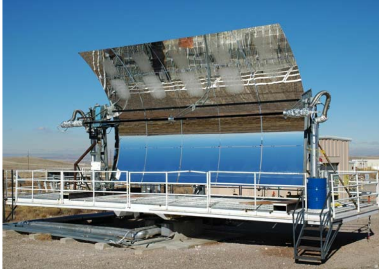
Figure 1: Picture of the LS-2 concentrator with the Schott HCE on the rotating platform at the NSTTF. The top two rows of mirrors still have the early morning frost.
