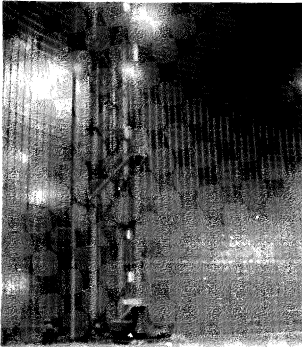
Figure 1.2.2-1 Technigaz Liner in Liquid Natural Gas Tank
