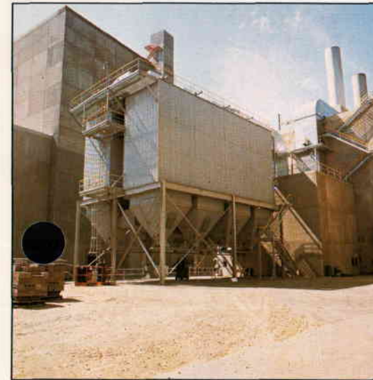
A power boiler fabric filter installation
