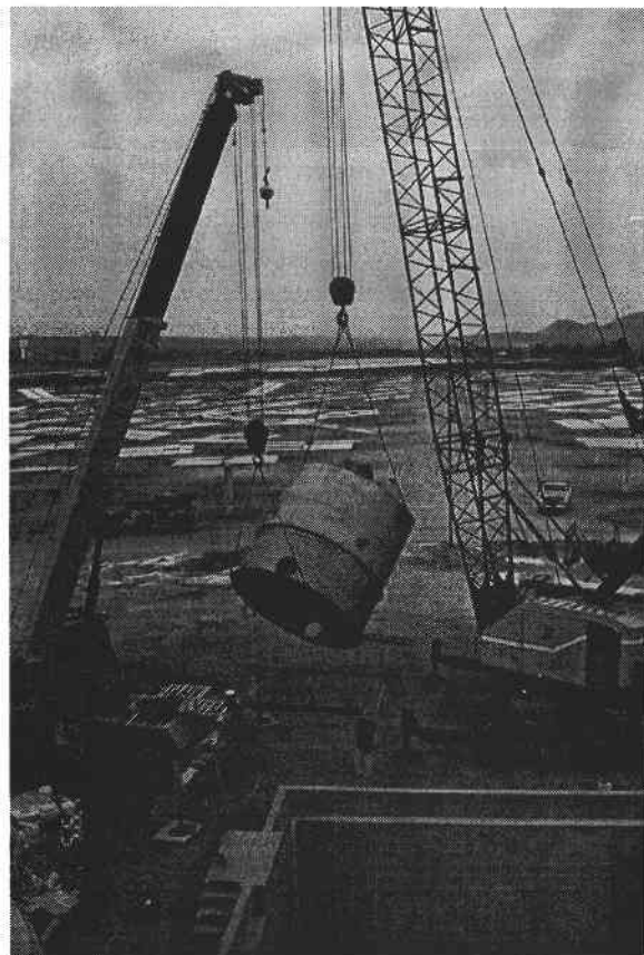
Figure 3. Installation of the pump sump for hot salt. Salt will be pumped from this vessel to the steam generator system.
