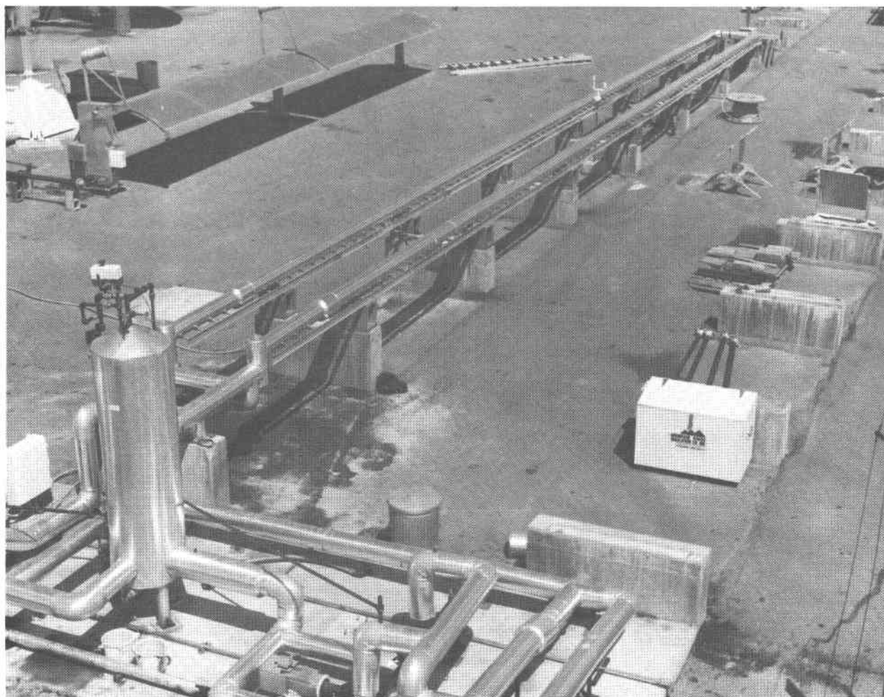
Figure 3-7. Heat Loss Test Loop at the Midtemperature Solar Systems Test Facility
