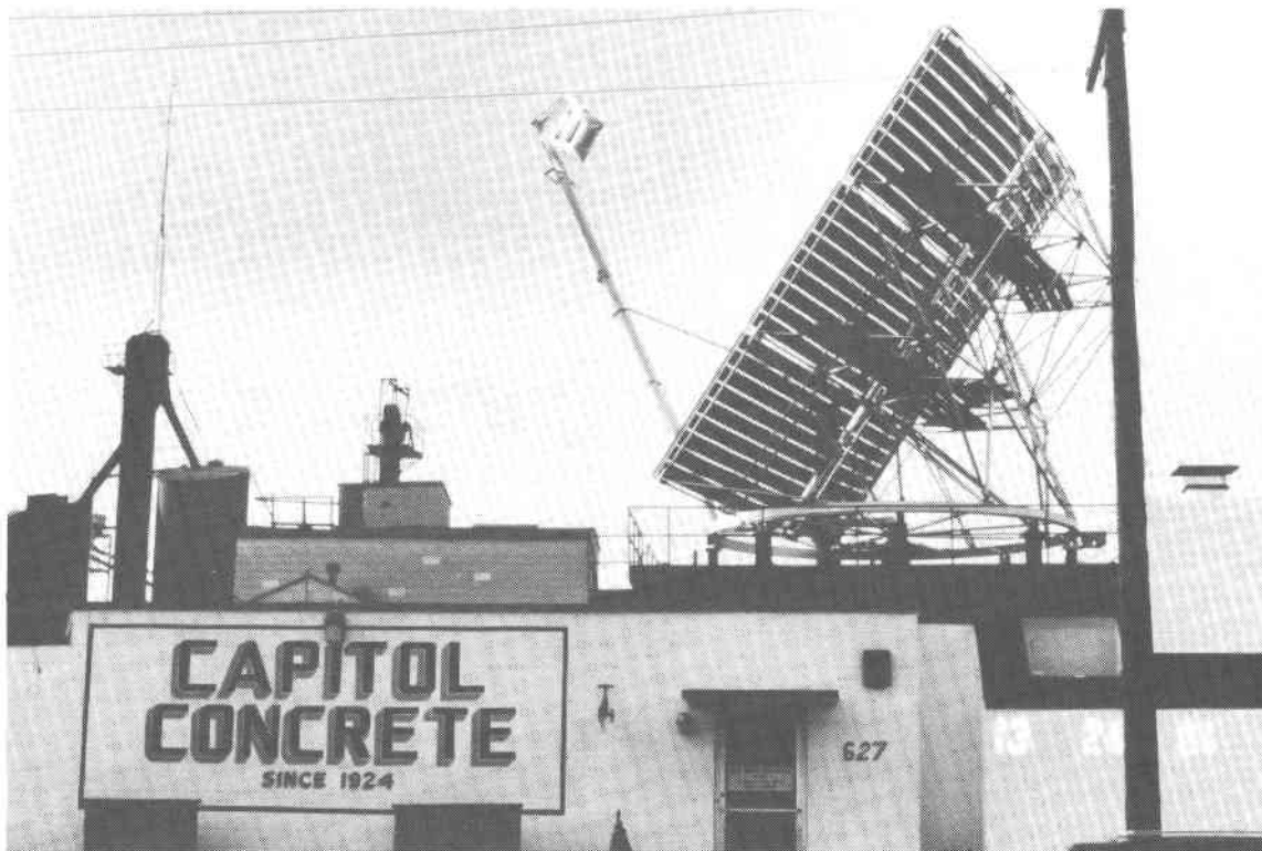
Figure 9. Power Kinetics Collector Installed at Capitol Concrete Products
