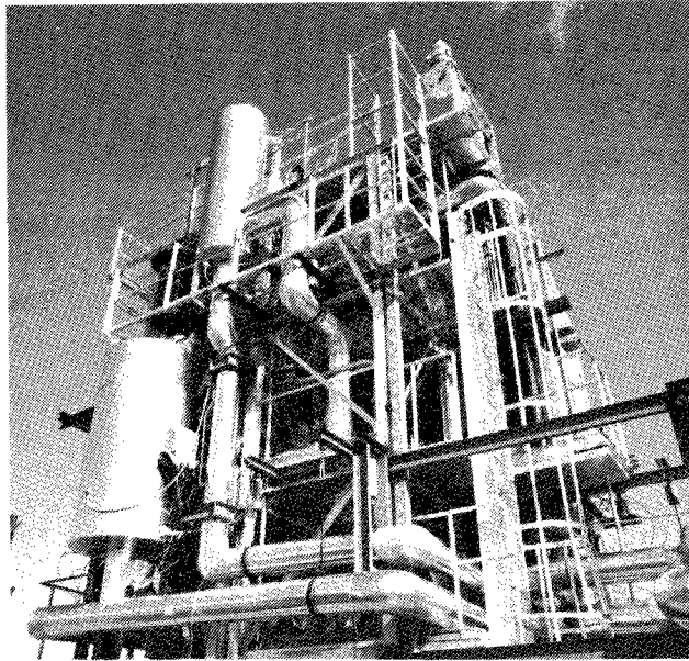
Figure 3-4. Exposed Receiver (South Side)
