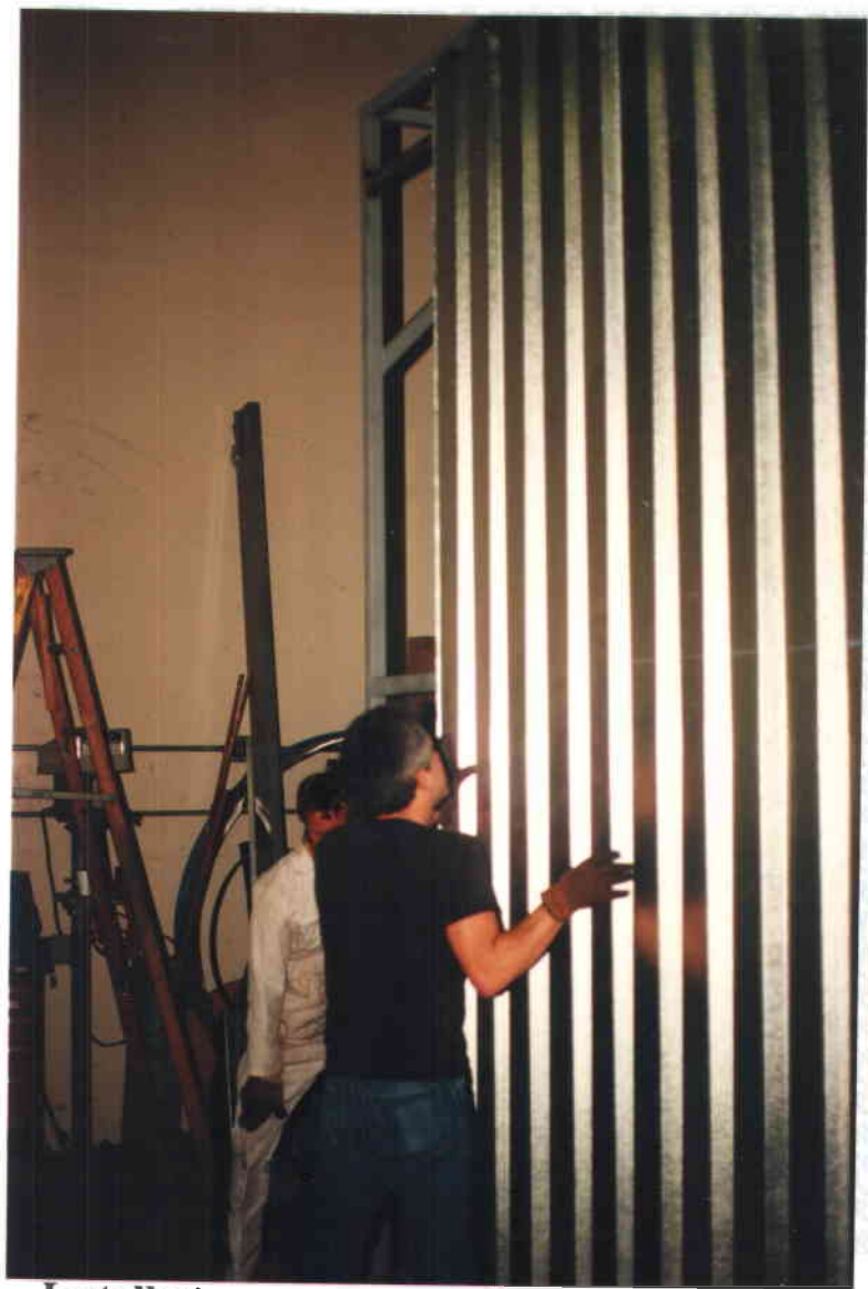
Installation of outer shipping container skin. Since the shipping containers are also designed to act as storage containers, they are sheathed with corrugated galvanized steel panels.
