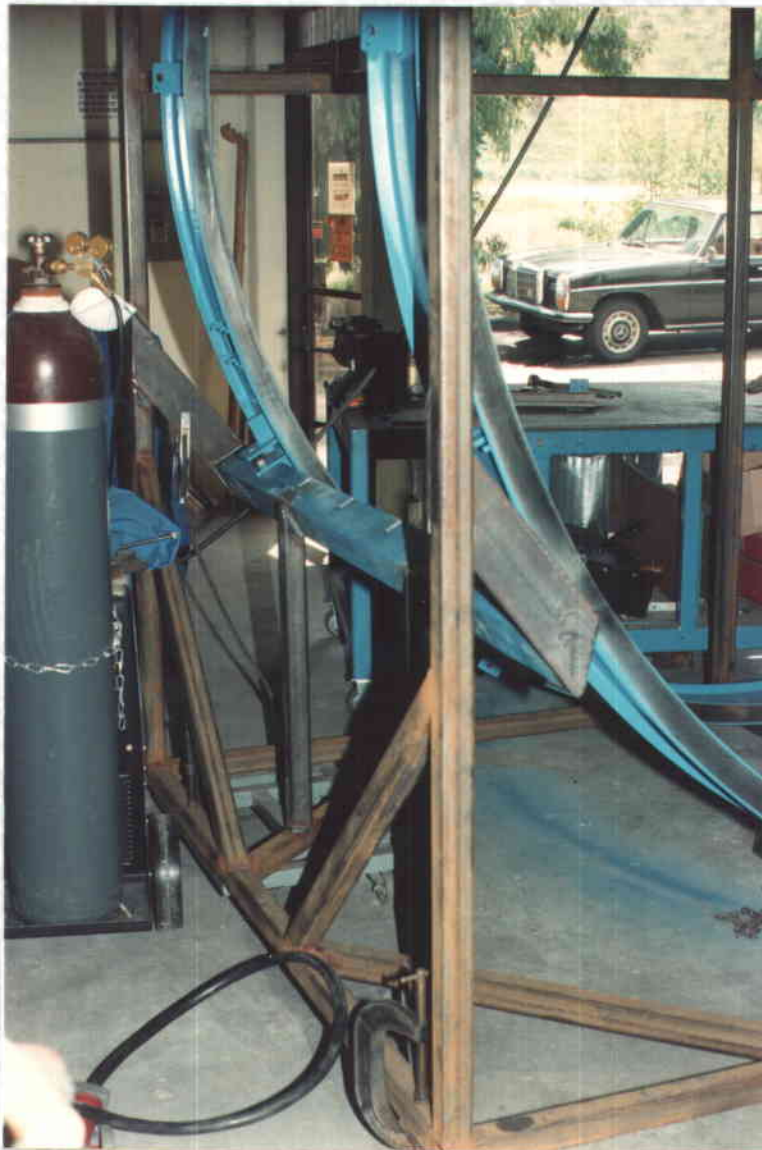
Welding of facet support rail assembly. The facets are mounted in the shipping container by their three mounting brackets. The two bottom brackets are mounted on side rails to support the weight of the facets.
