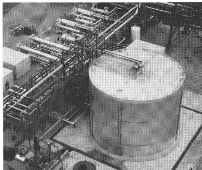
Figure 4.15. Solar One's Mixed-media Thermal Storage Unit
