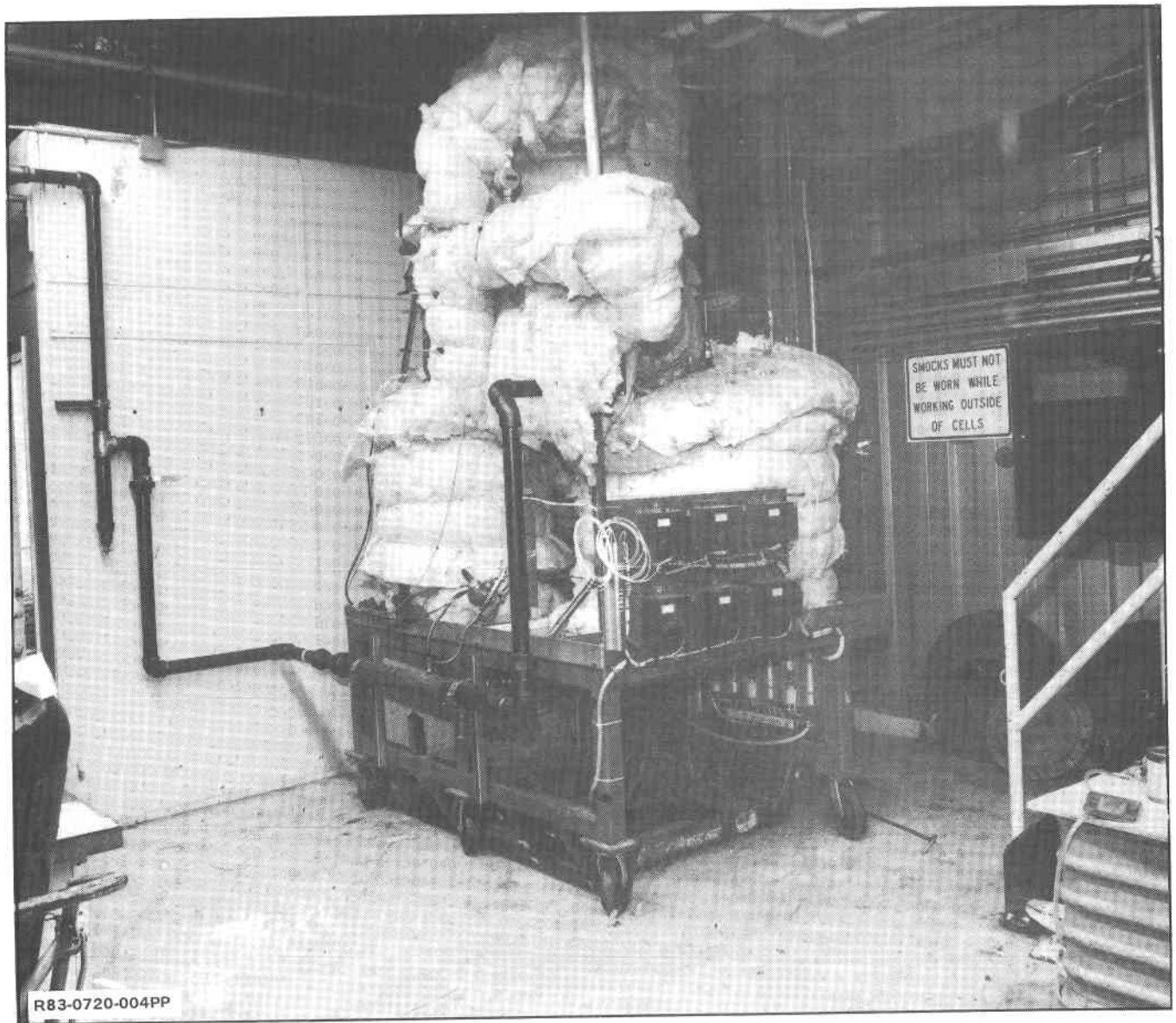
Fig. 2-3 Direct-Contact Heat Exchanger, Refurbished System
